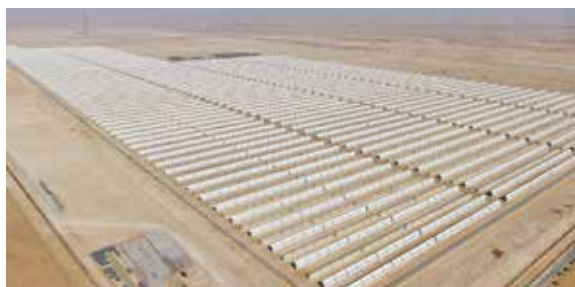
Dubai's concentrated solar thermal power plant
